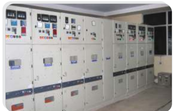
11kV VCB Panel
